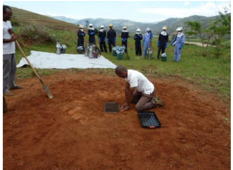
Installing a Mobile Soak Pit to adsorb and safely degrade the traces of insecticide found in the wash-water.
